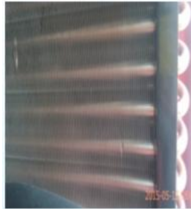
2. This is a condenser (the copper pipe of the condenser in the figure is horizontal and the fin is vertical)
